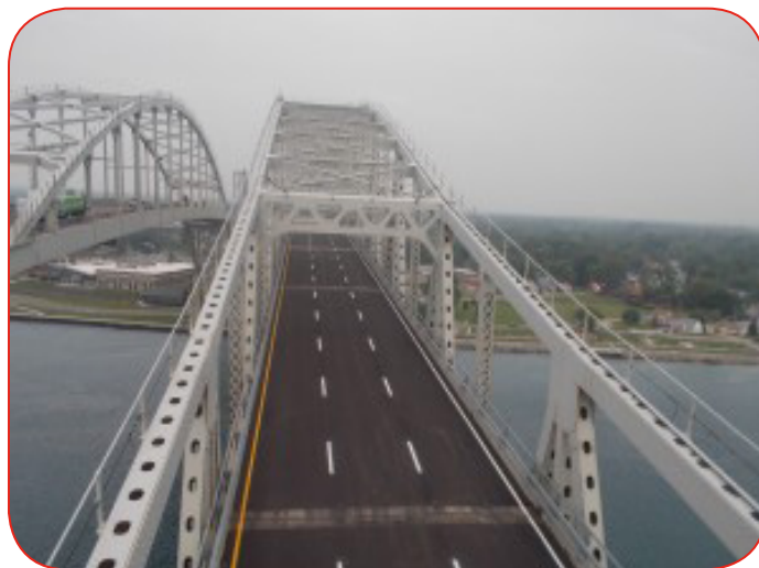
Aerial view of the Blue Water Bridge Canadian and U.S. bridge spans in Point Edward
