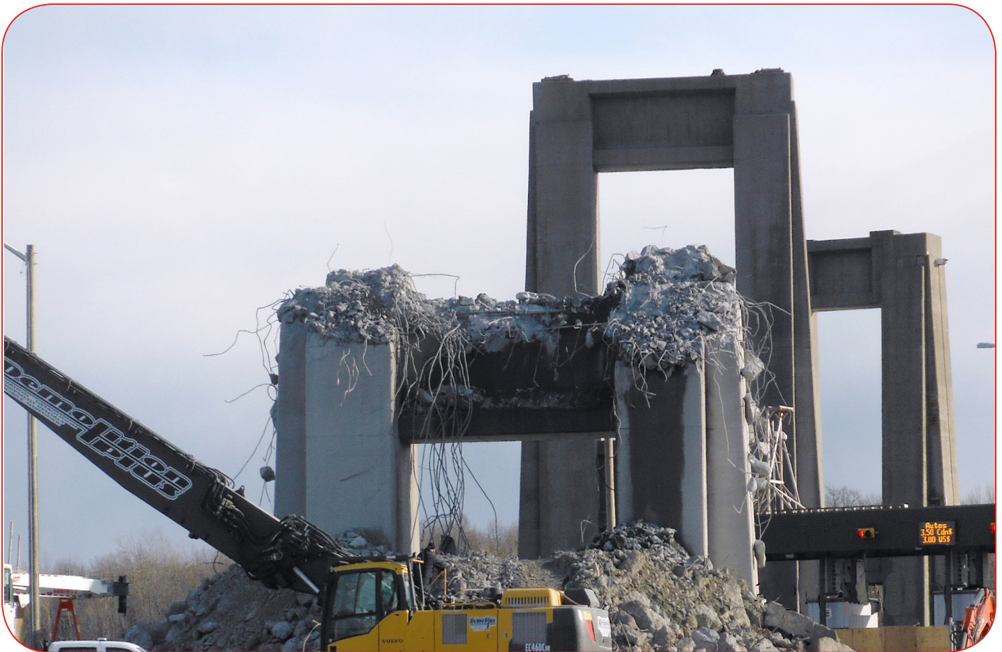
Toll collection in operation while the final phases of the North Channel Bridge demolition is underway at the Seaway International Bridge in Cornwall
